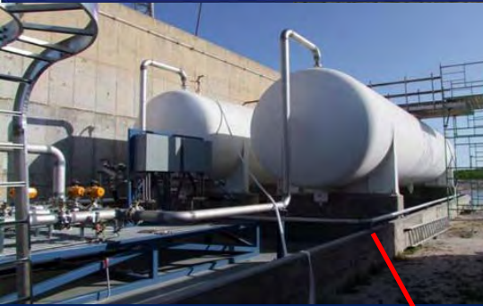
RP-1 Fuel Tanks & Skids
